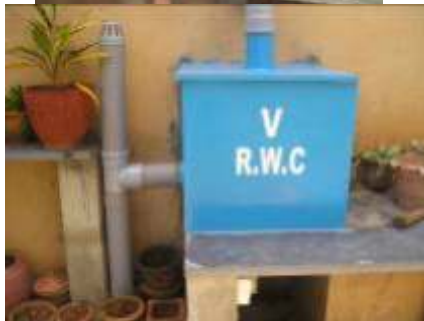
Ferro cement filters
