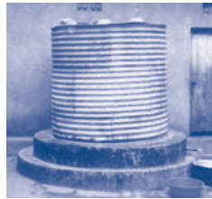
A corrugated steel tank in rural Uganda. Note the darker ring at the bottom of the tank – a concrete repair that is often needed (Picture: D. Rees)
