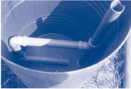
Pipe arrangement for sand filter
