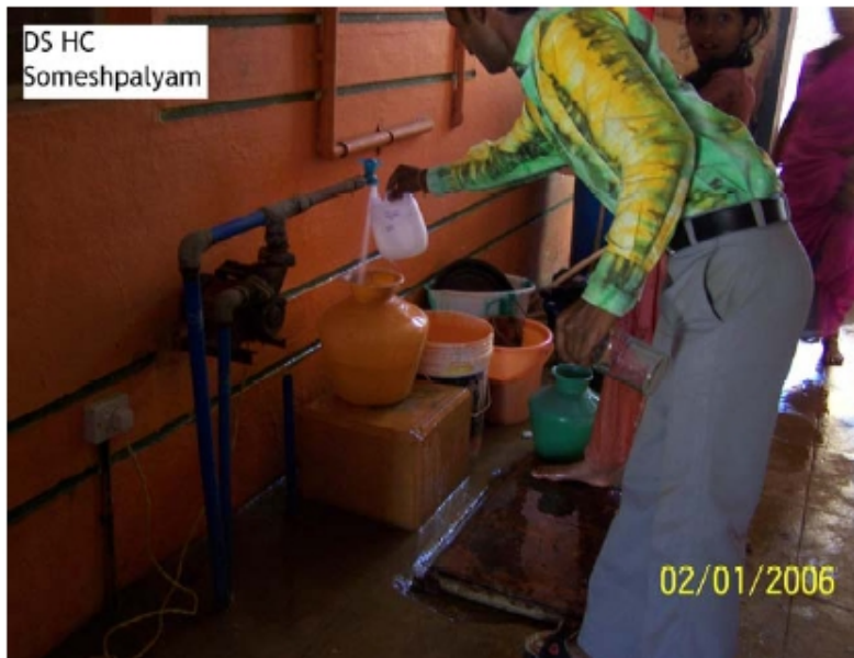
Figure 10: Water supply point at individual household (inside town) supplied by Someshwarapalya reservoir
