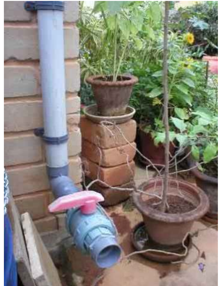
First rain separator with gate valve
