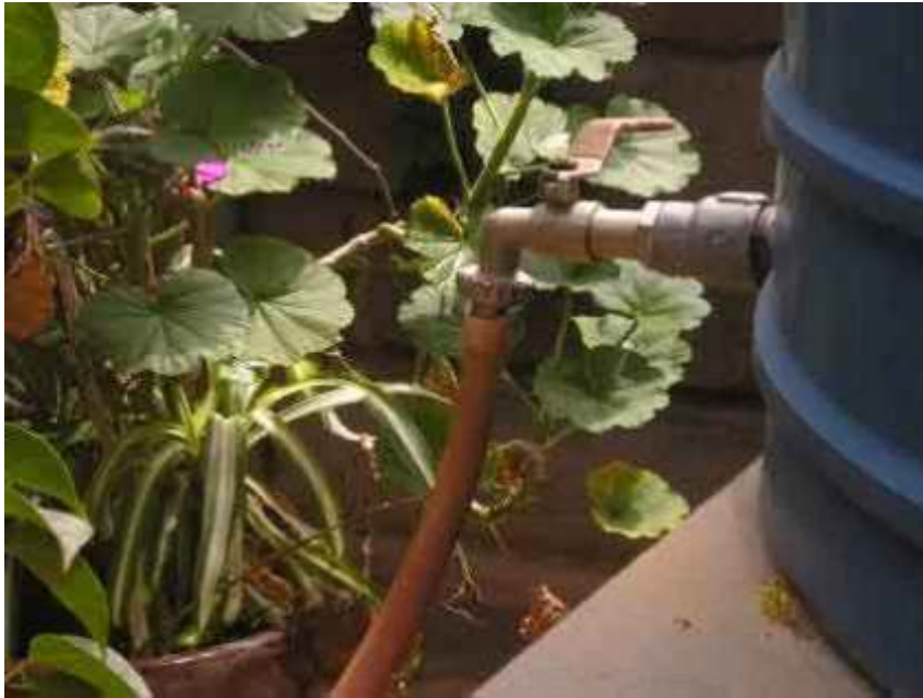
Using a hosepipe, the tap can be connected to the borewell or sump tank.
