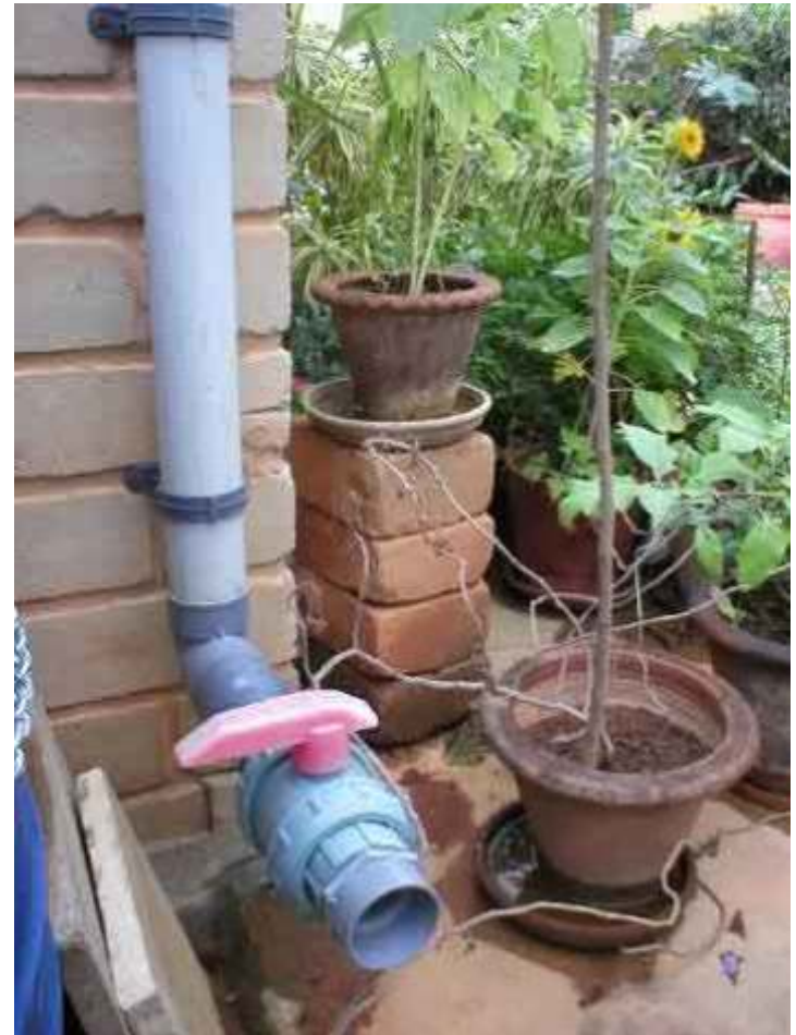
First rain separator with gate valve
