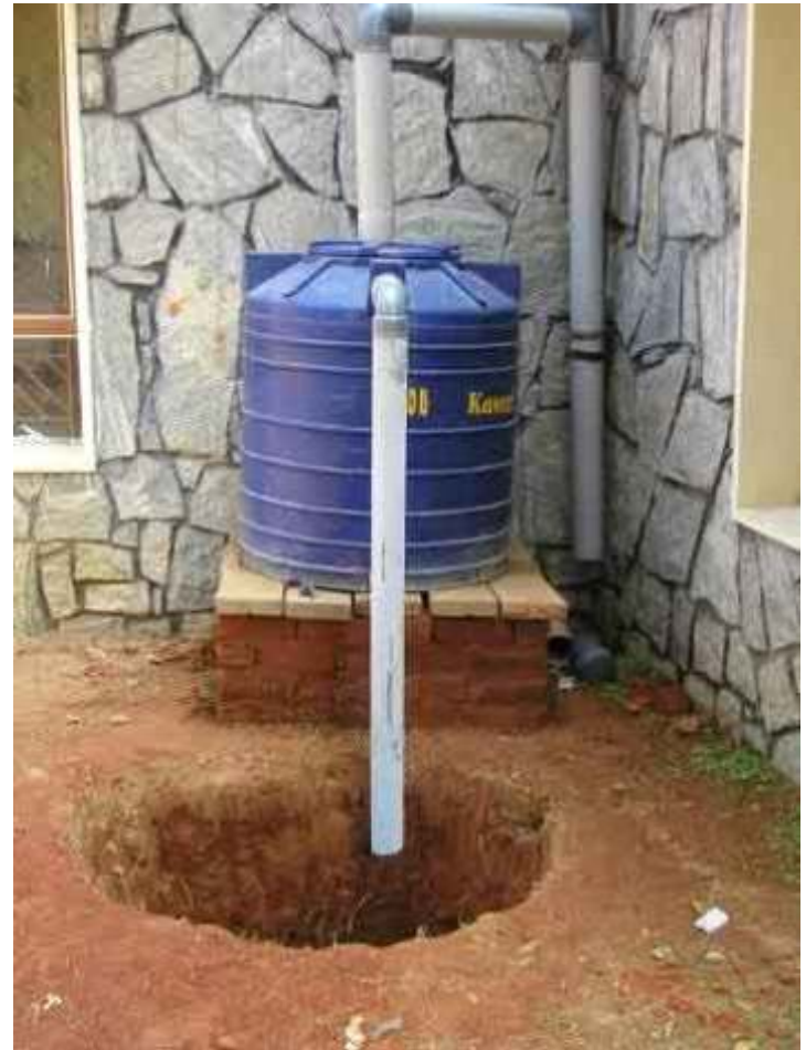
Overflows from rain barrels can also be used for recharging the groundwater
