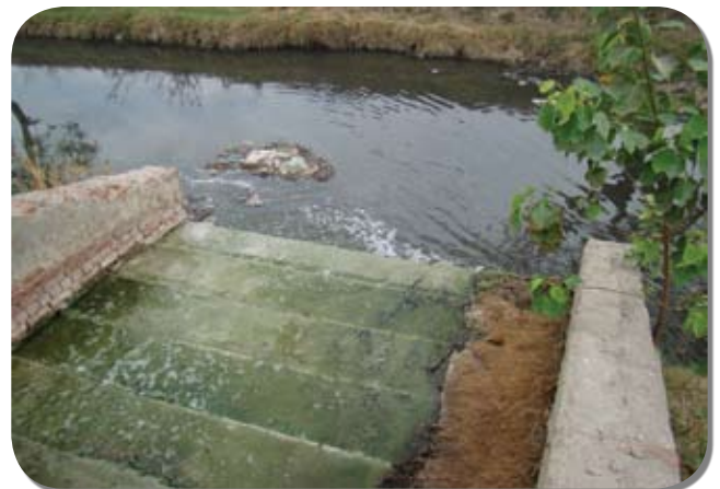
Pic 16: Treated effluent from 30 MLD STP at Sonapat is falling into the polluted waters of Drain no 6. (16.6.10)
