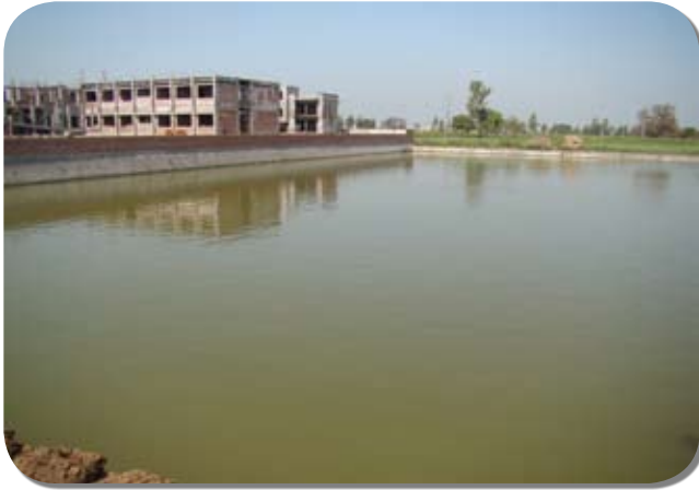
Pic 23: Hospital (36 bed) under construction in part of the village pond land (Daclana village). 12.4.10
