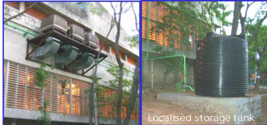
Modular spot coolers used for shop cooling
