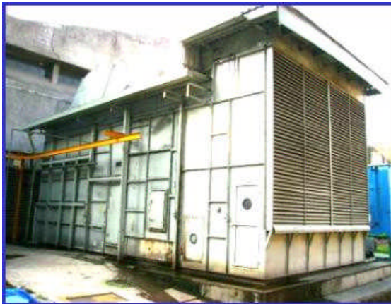
ARP was used for shop cooling
