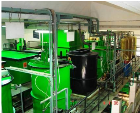
EFFLUENT TREATMENT PLANT
