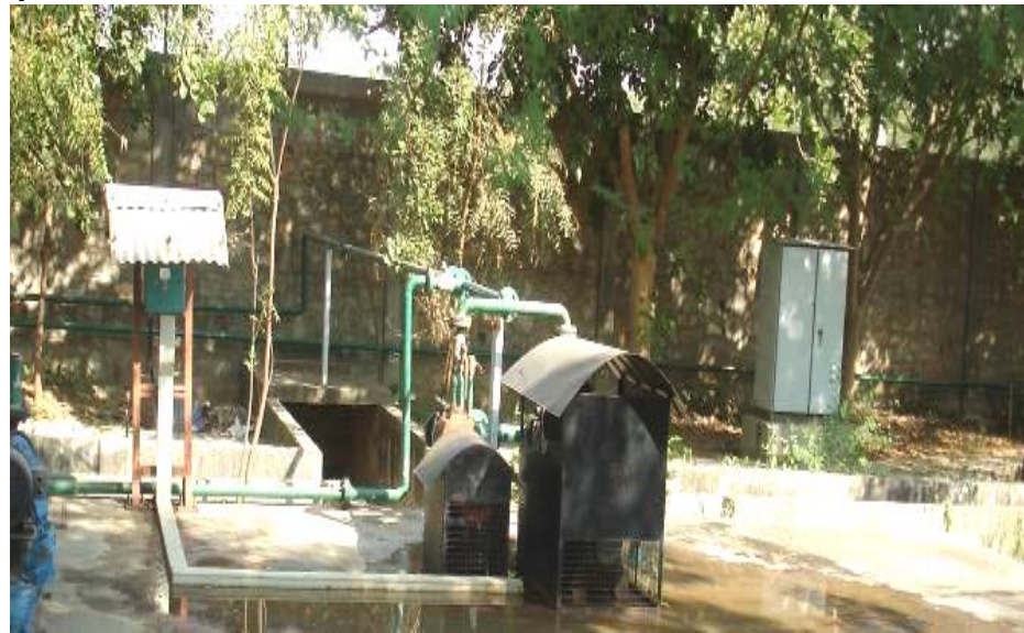
Pumps and collection system
